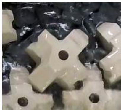
Figure 3.4: Failed unit at position that facilitates rocking
