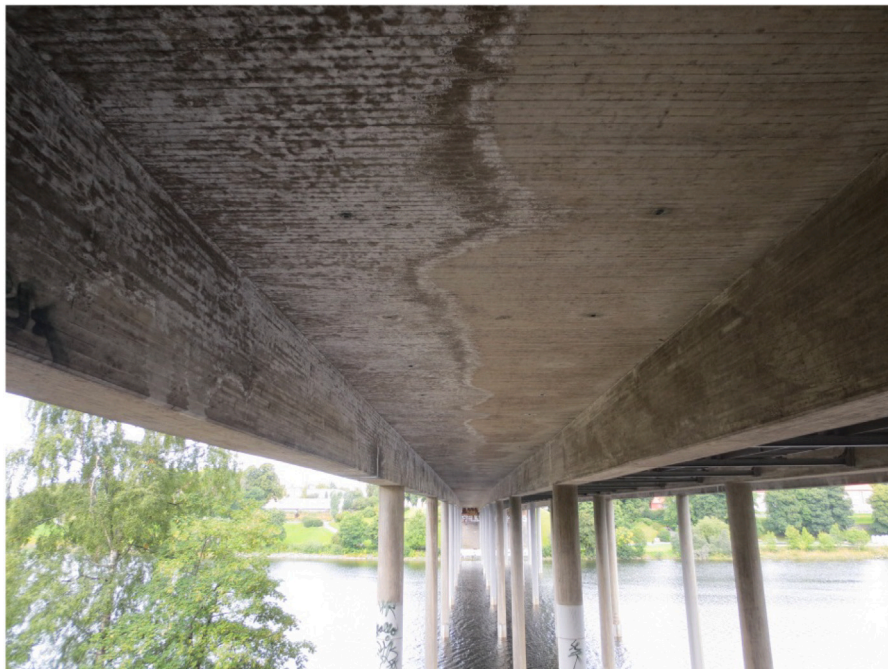
Fig. 7. There is a sign of water penetration of the bridge deck in outermost region of the bridge. The image shows the western outer and western inner beam. Image courtesy of Dr. Ing. A. Aas-Jakobsen AS.
