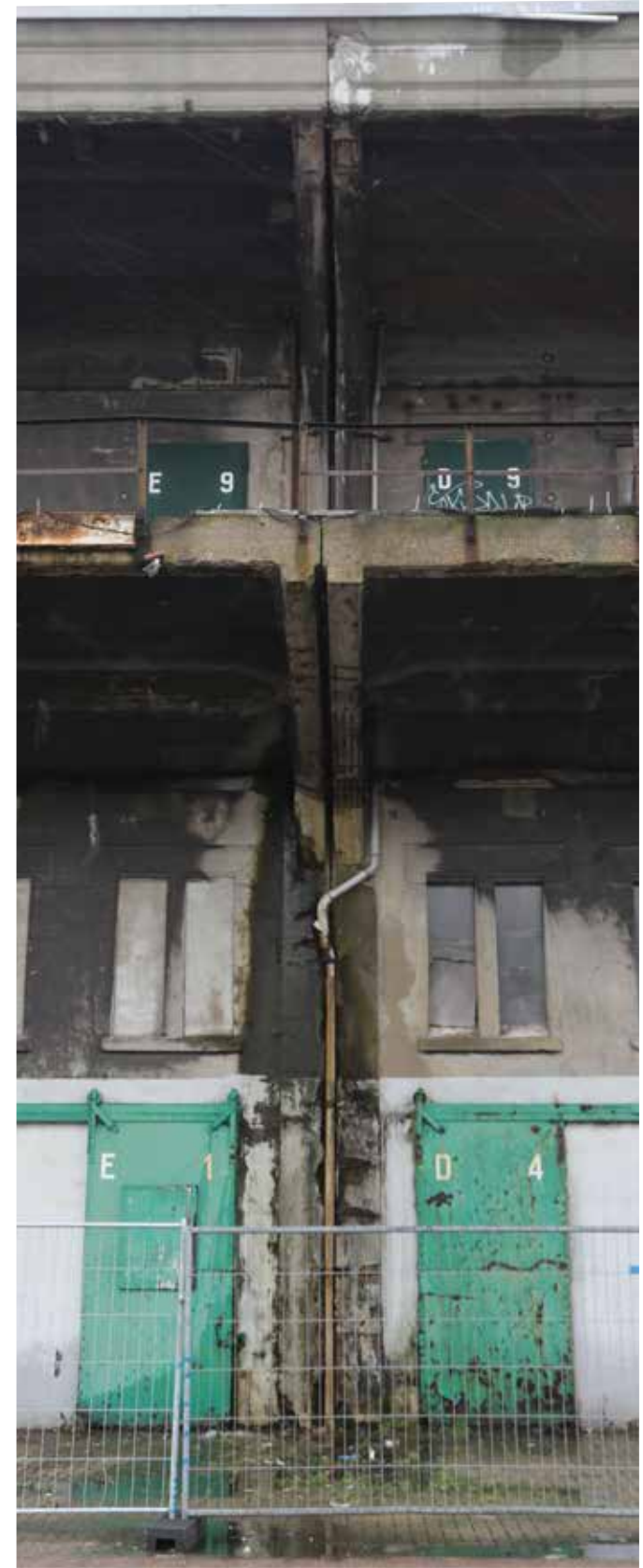
Exterior in bad condition, building no longer in use
