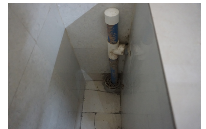
Figure 18: The drain in hospital 2.
