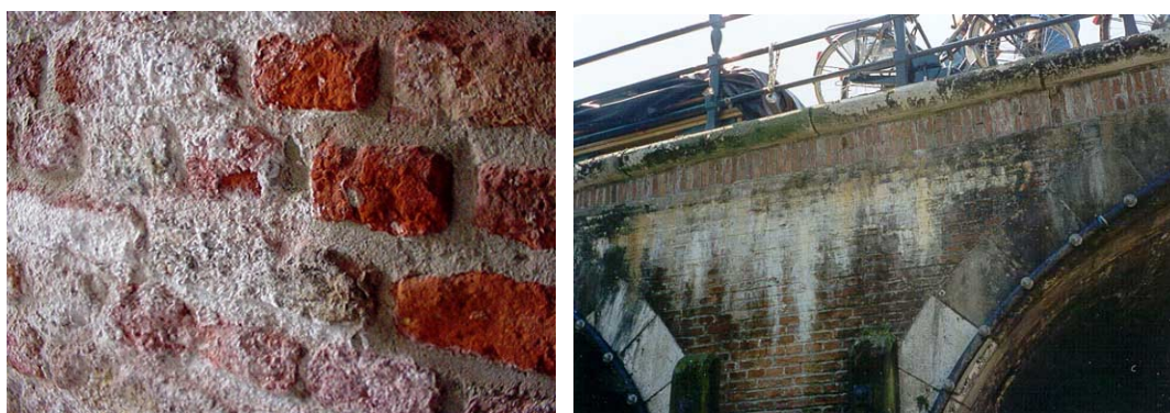
Figure 2: Salt efflorescence (l) and encrustation due to leaching of mortar constituents (r)
