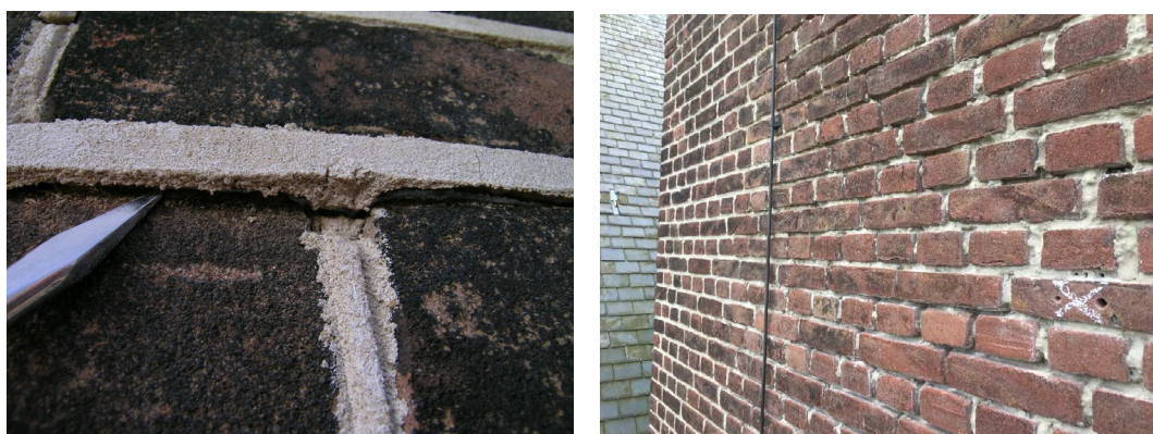
Figure 3 Examples of push out of pointing(l) and erosion (r)
