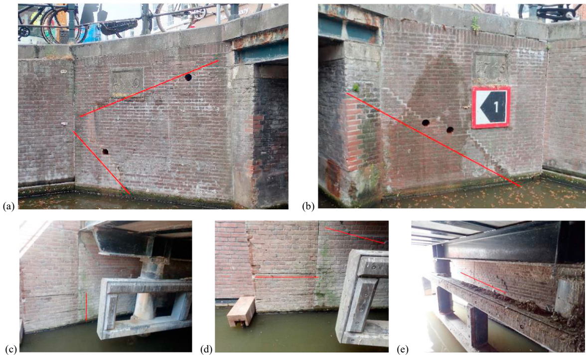
Fig. 2. Diagonal cracks in the West (a) and East (b) wing walls. Vertical (c) and horizontal (d,e) cracks on the East abutment.
