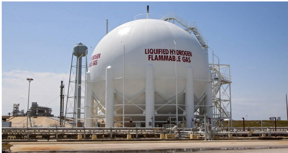
Figure 6.26: A liquid hydrogen storage tank (NASA, 2015).
