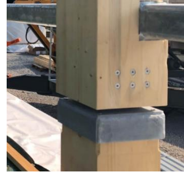
Figure A-35: Connection between columns (B&O Wooden Multi-Storey Car Park, Bad Aibling, n.d.)
