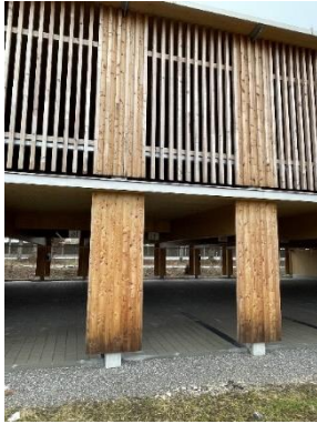
Figure 12-1: Wood protection panel
