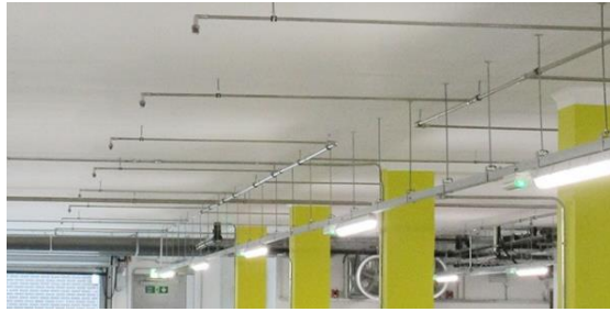
Figure 5-5: Sprinkler system below the ceiling (Martinez, n.d.)
