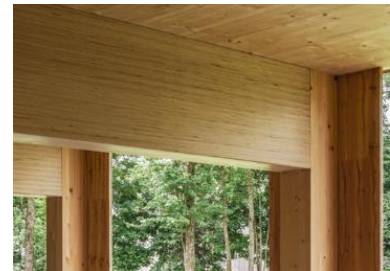
Figure A-37: Connection between timber beam and column level 1 (B&O Wooden Multi-Storey Car Park, Bad Aibling, n.d.)
