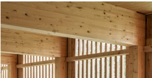
Figure A-36: Connection between timber beam and column level 2 (B&O Wooden Multi-Storey Car Park, Bad Aibling, n.d.)
