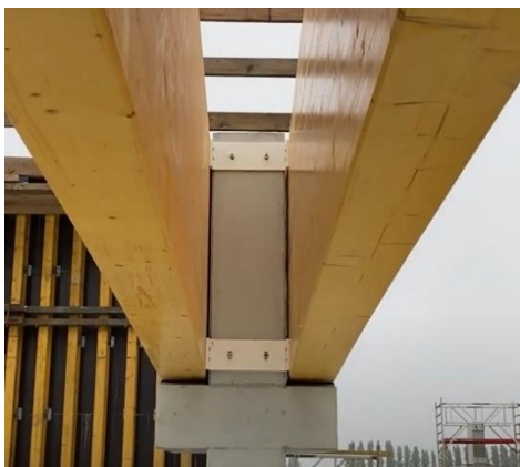
Figure A-4: Connection between timber beams and column ( Oosterweel Verbinding: Hout En Beton Op Park & Ride [Powerpoint-Slides], n.d. )
