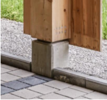
Figure A-34: Connection foundation to column (B&O Wooden Multi-Storey Car Park, Bad Aibling, n.d.)
