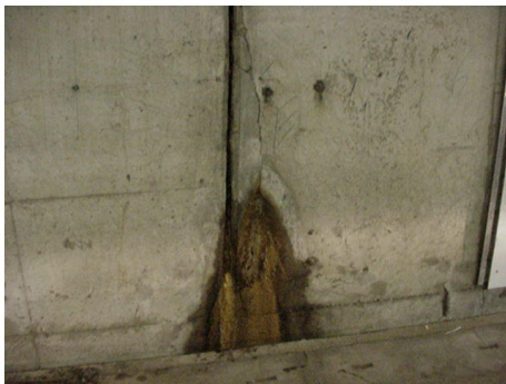
Figure 1.6: leaky joint with crack situation in 2001
