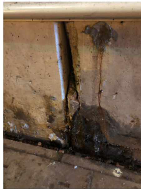
Figure 1.7: leaky joint situation in December 2019
