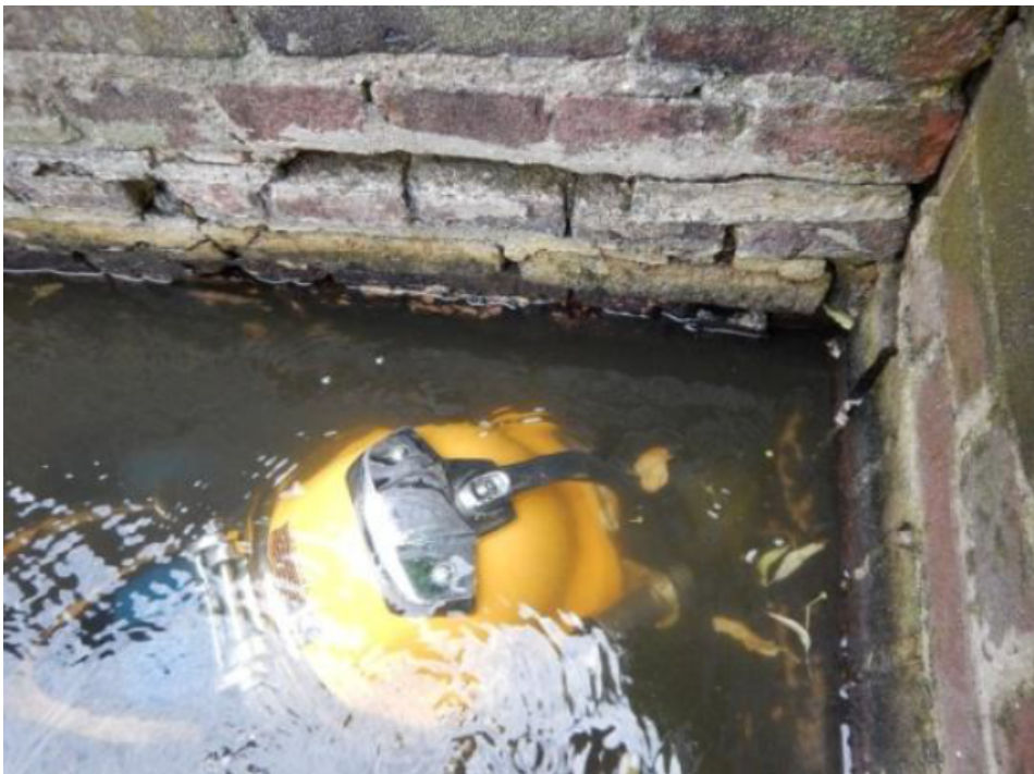
Figure C.5: At the water line large quantities of the mortar has washed away. A number of bricks are no longer connected to the quay wall, other bricks are missing. The pores which were created by the washed away mortar have an average depth of 40 mm , with maxima up to 100 mm .
