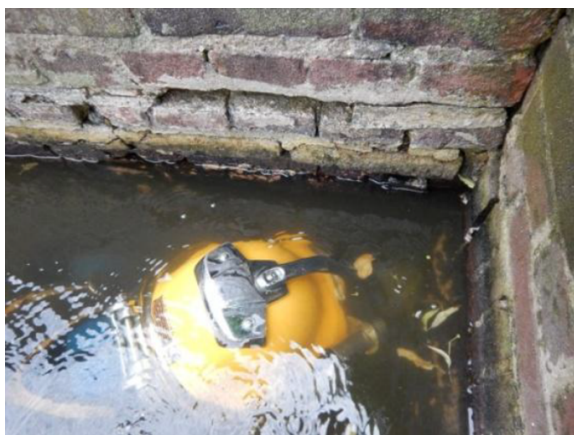
At the water line, large quantities of the mortar has washed away. A number of bricks are no longer connected to the quay wall, other bricks are missing. The pores which were created by the washed away mortar have an average depth of 40 mm , with maxima up to 100 mm .
