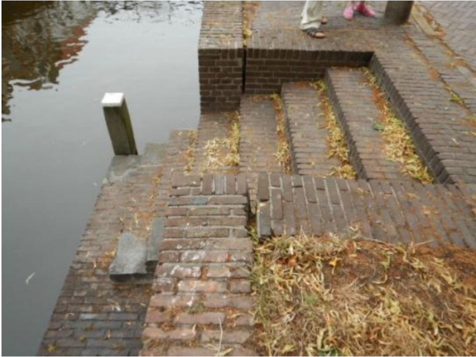
Figure C.2: The front side of the quay wall has settled more than the quay and street, resulting in a small inclination. At the location of this picture the horizontal displacement is 65 mm .
