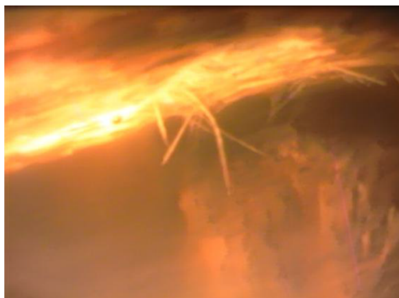
At various locations the piles of the front row are no longer connected to the capping beam above it. Wood-decay is deemed as the cause for this. This space ranges from 30 mm up to 150 mm .
