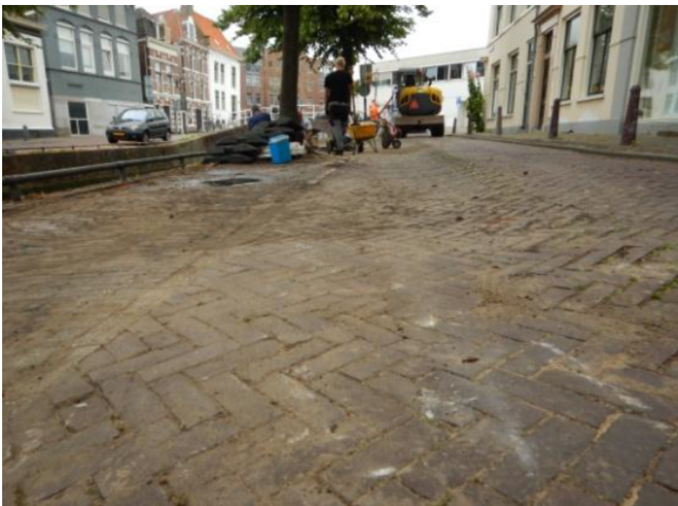
Figure C.1: Settlements are observed at multiple locations on the upper side of the quay and the street connected to it, indicating settlements of the subsoil.
