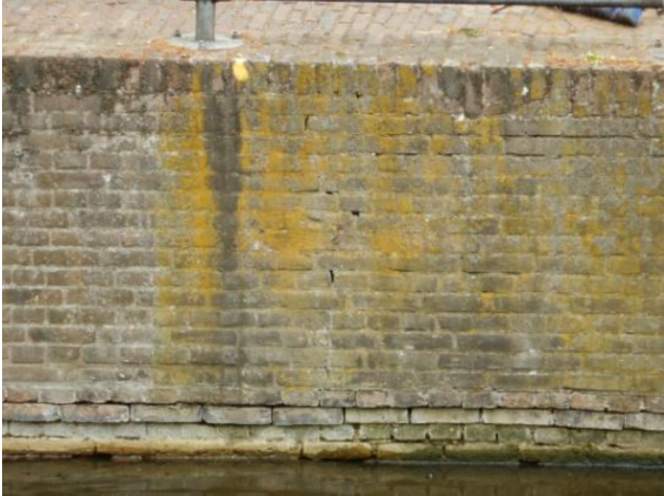
Figure C.4: The masonry of the quay wall has deteriorate over its full length. At various locations the mortar has been washed away and cracks have formed over the height of the wall. The bricks are cracked as well.
