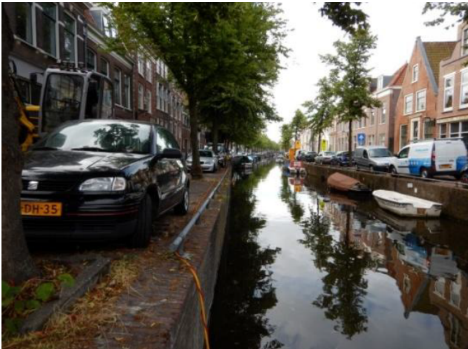
Figure C.3: Over the full length the quay wall bulges towards the channel.
