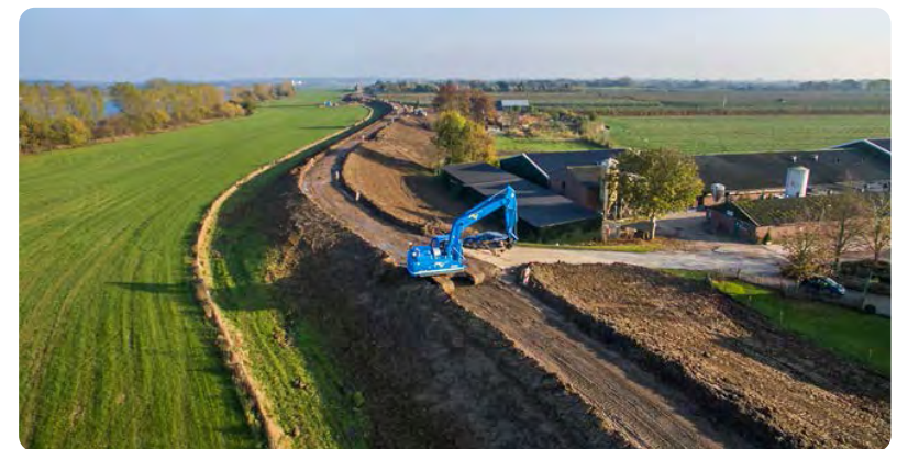
Figure 1: Construction of a dike. Source: HWBP (2018, p.103) , photo taken by Pascal Ogink.
