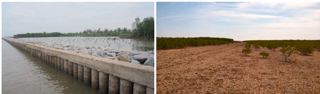
Fig. 8. (a) Existing coastal protection structures, (b) Groynes systems in Camau, (c) Mangrove restoration project in BacLieu.
