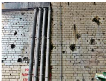
World War II shrapnel damage still visible underneath Blackfriars Road rail bridge
