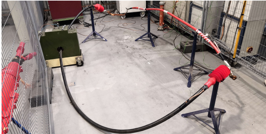
Figure 6.18: Reference cable testing setup.
