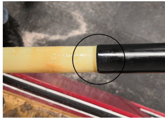
(b) semi-conductive screen interruption inside the joint.
