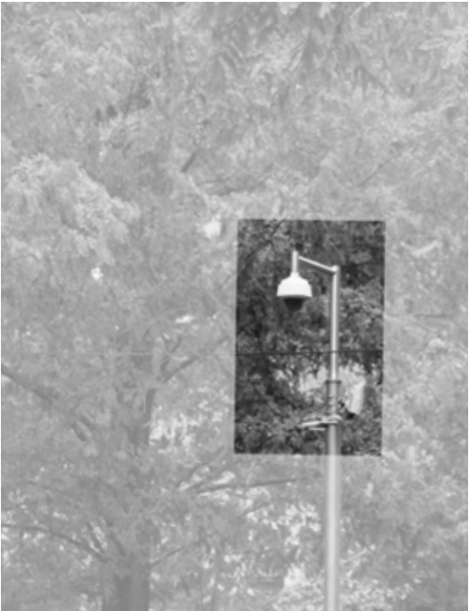
Jubilee Park CCTV Maintenance and safety elements
