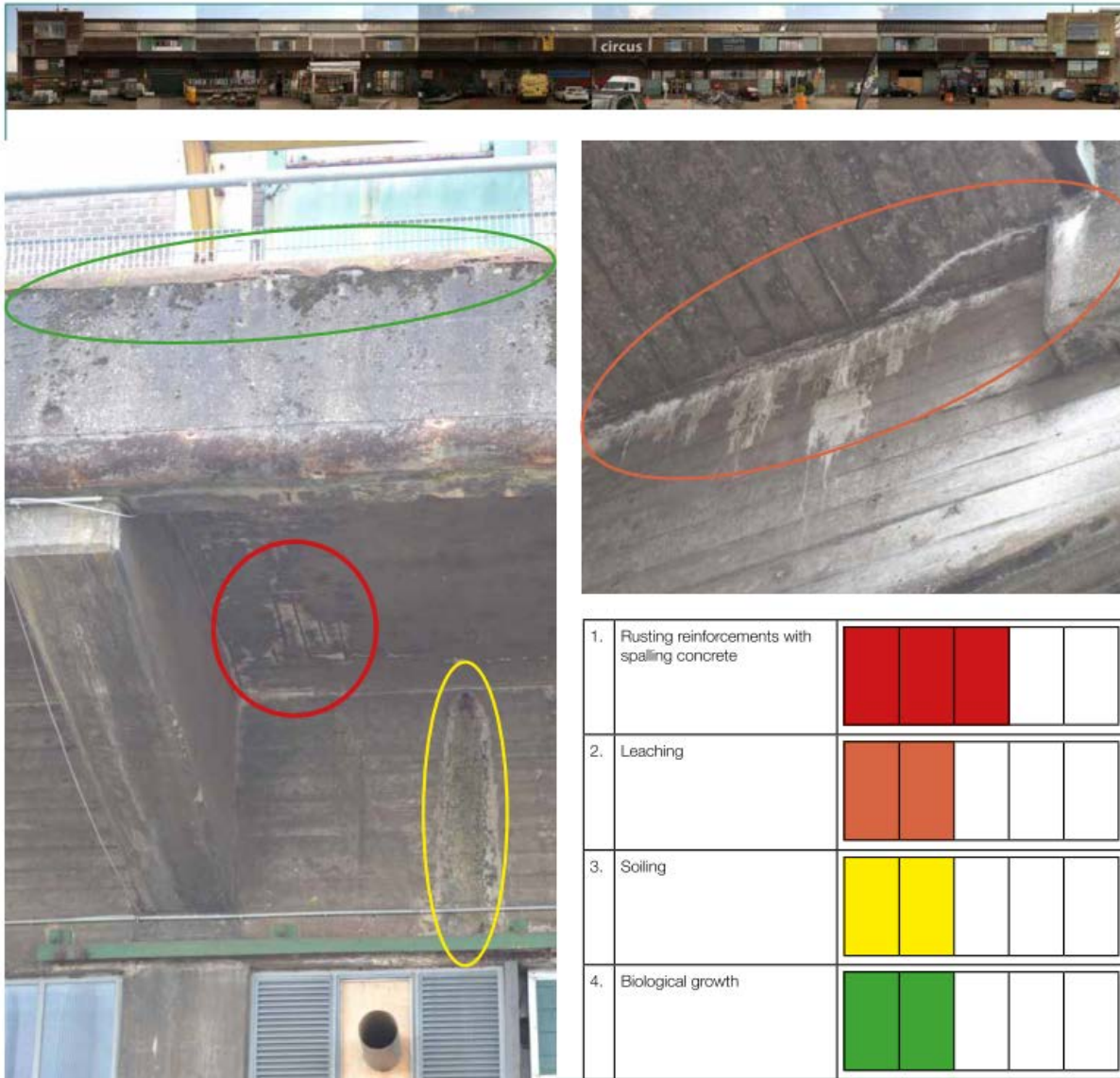
Figure 31 - Damages North facade - Own Illustration
