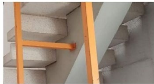
stairs of white and pale artificial stone bear off on concrete stair-beams
