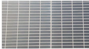
glazed brick slabs in tile pattern (glued on concrete prefab panels) exterior
