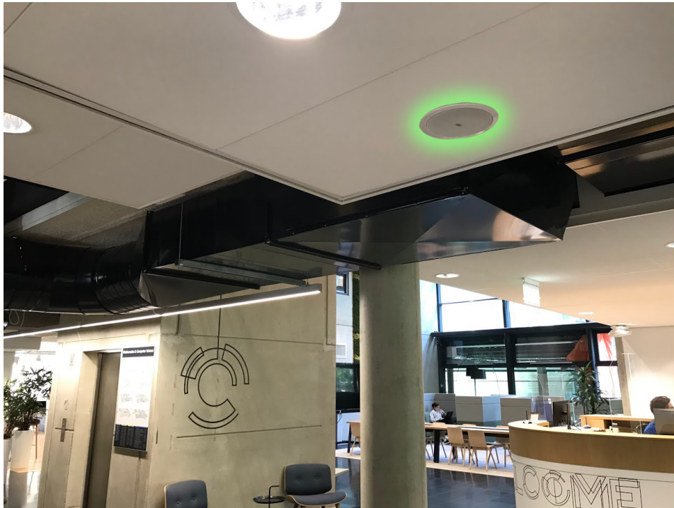
Figure 2.1: An example of a PA system speaker integrated into the ceiling (indicated in green).
