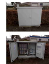
Street junction box Bijvank Glasvezeltechni- et, n.d.
