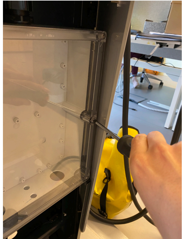
Figure 69 & 70. The side panels obstruct the installerbox lid. ▼ ▲
