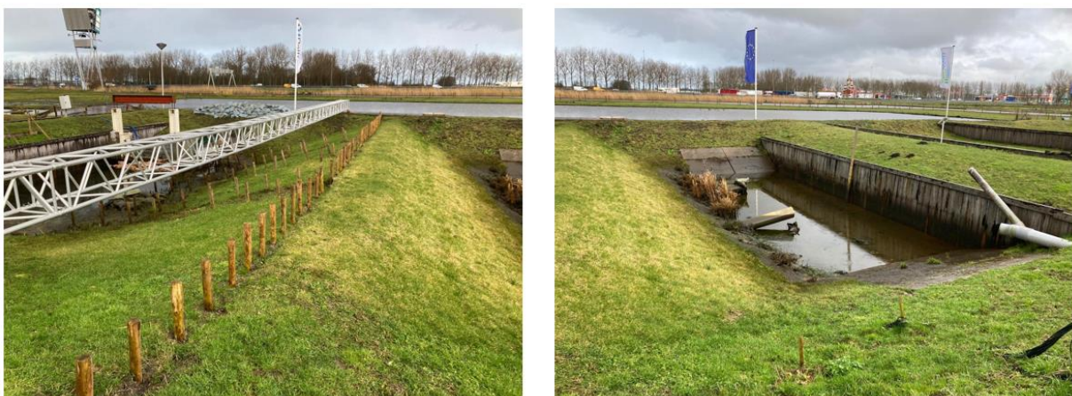
Figure 35: State of dike before physical tests
