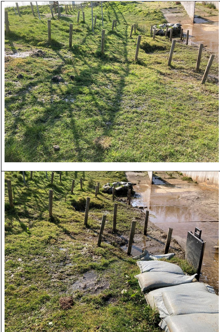
Figure 80: Inner slope of dike where water is present at the dike surface directly above the tube with sliding door
