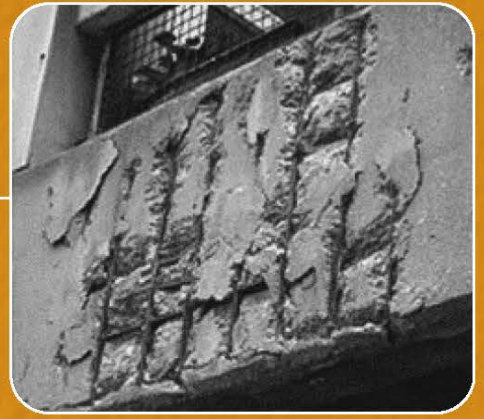
Damage to Free Surface of Element
