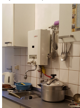
Fig. 1.2.7: Family: Gasboiler (open geiser)
