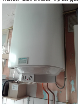
Fig. 1.2.5: Student 4: Electric boiler
