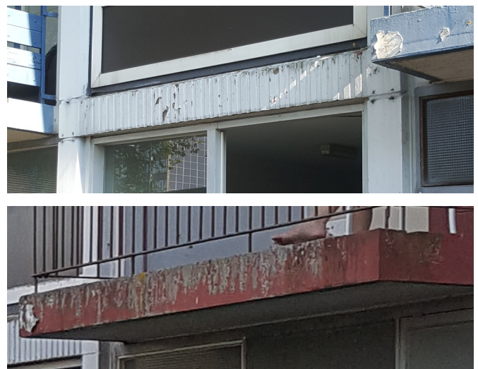
Figure 1.3.6 . Cladding with poor maintenance
