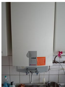
Fig. 1.2.2: Student 1: Gas boiler
