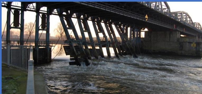
Figure 3 Aftermath of ship collision with the weir at Grave. Source: Rijkswaterstaat
