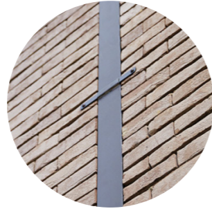
Aluminium rainwater pipe
