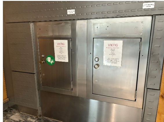
Figure 12: Hatches of the vacuum system that was used in the past for waste transportation at Oslo Airport. (Own figure).
