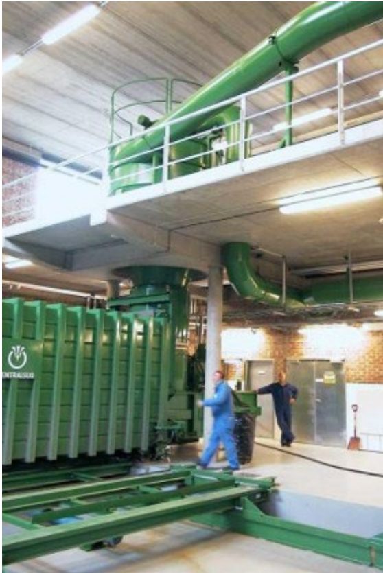
Figure 11: The endpoint of the vacuum system that was used in the past at Oslo Airport for waste collection and transportation (Avinor Oslo Airport, 2024)
