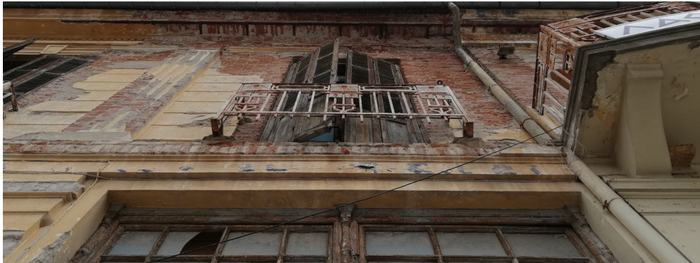
Figure (70) : Destroyed façade, worn off plaster _Soith-West Facade (Survey Document) (Personal Document)
