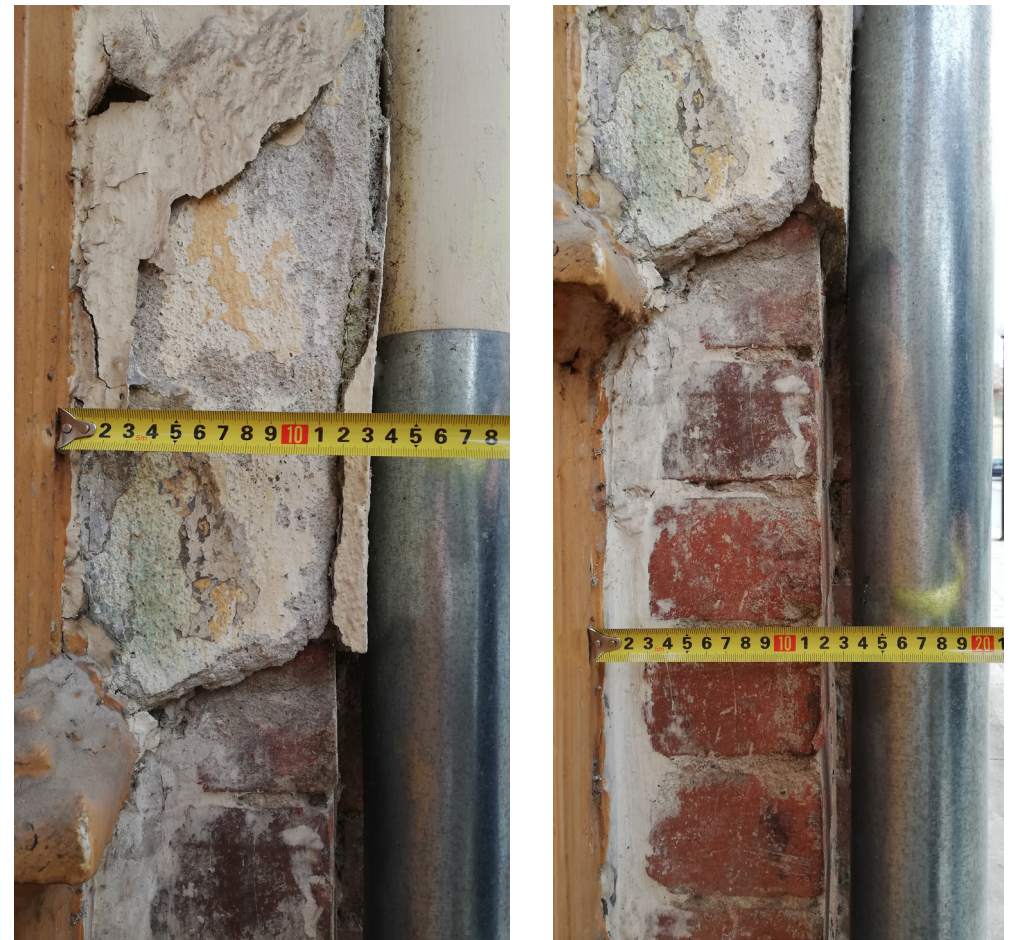
Figure (68) : Destroyed façade, worn off plaster detail_North-West Facade (Survey Document) (Personal Document)
