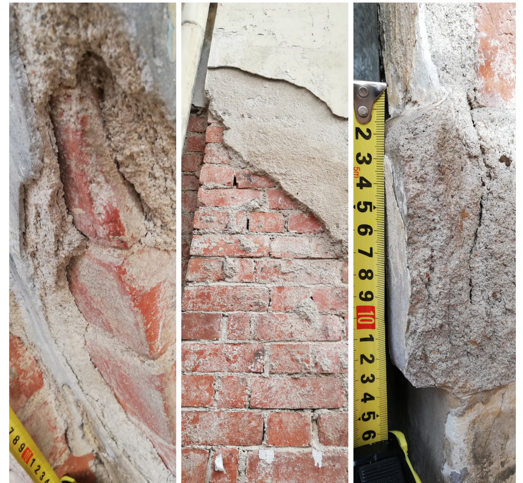
Figure (71) : Plaster damage on south-west facade (survey product)
