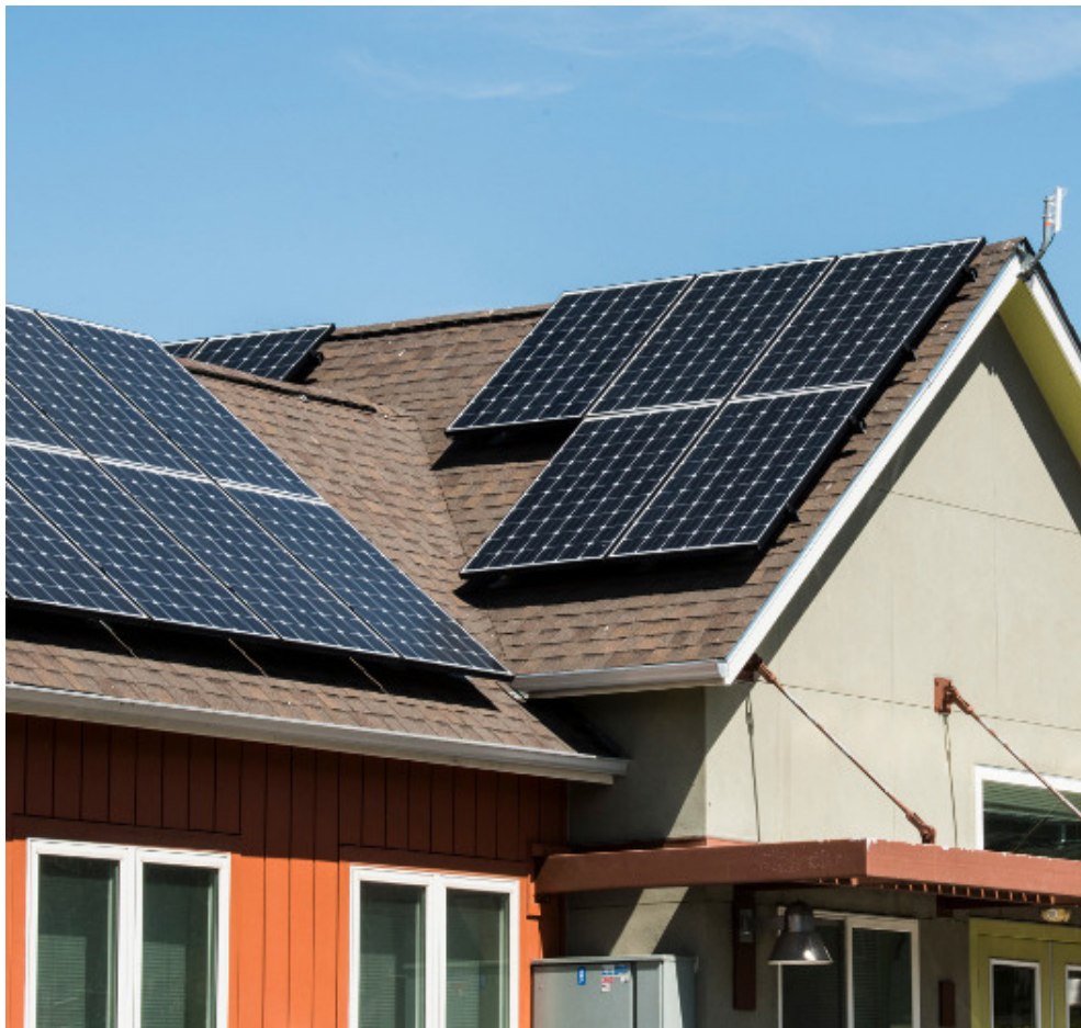
Figure (9): Photovoltaic modules on roof ( http://slapcoffee.com/ )
