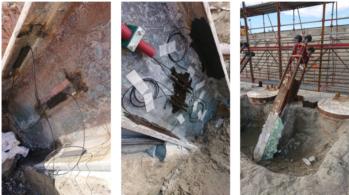
Figure 4.4: Mounted FBG sensors on MV-piles A11, B4, B14, C2 and D1
