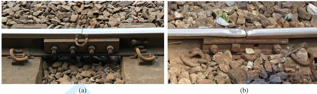
Figure 1. Two examples of rail joints: (a) invisible damage: loose bolts, and (b) visible damage: missing bolt and battered rail surface
