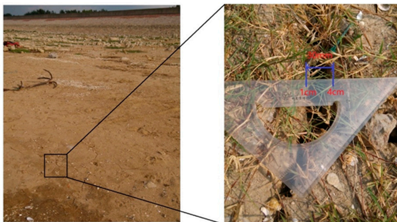
Figure 4. Cracks with maximum width of 30 mm on the upstream slope.
