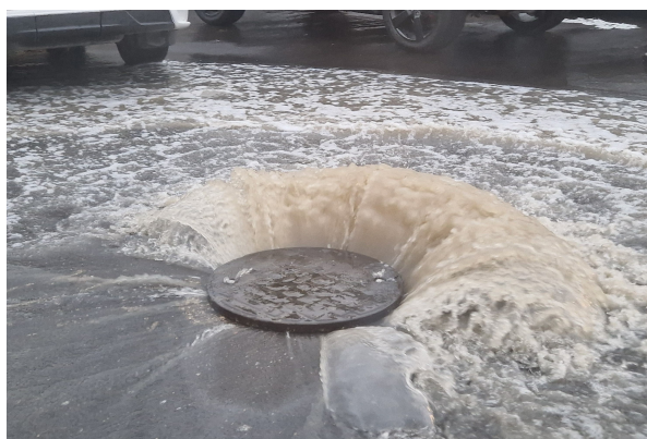
Figure 4.1: Image of an overflowing drainage gullie.
