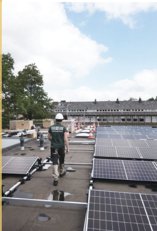
WijkEnergieWerkt employee on the solar roof being installed on Dalton school De Margriet
