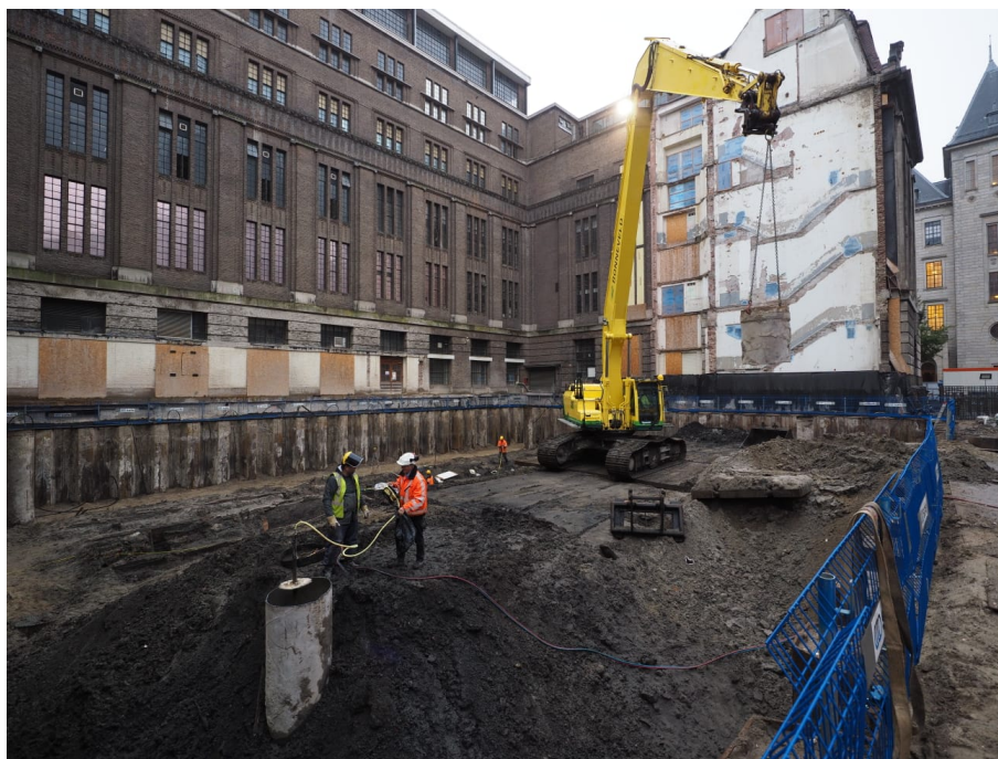
Figure B.3: Installation (and instrumentation) of screw-displacement piles. Excavation level at -2 m NAP is taking place.
