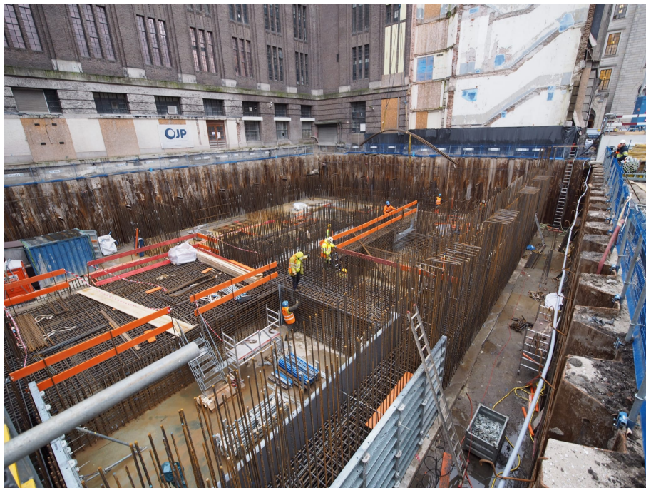
Figure B.7: Installation of reinforcement for future casting of basement and ground floor.
