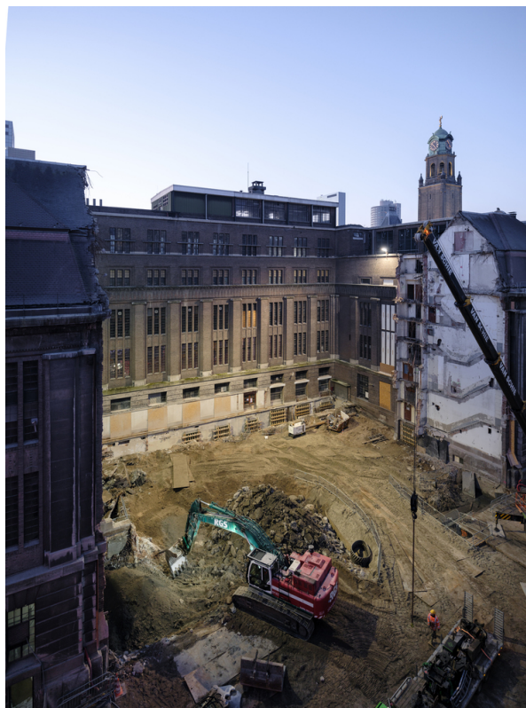
Figure B.1: Demolition of the existing wall adjacent to Rodezand street and preparation of the work site (from Arch Daily, 2023).
