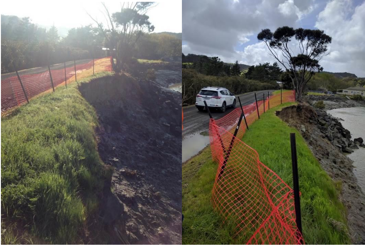
Figure 2: Access road erosion on the 9 th September and 3 rd October 2019. Approximately 0.5m erosion since the previous picture taken on 21st March 2019.
