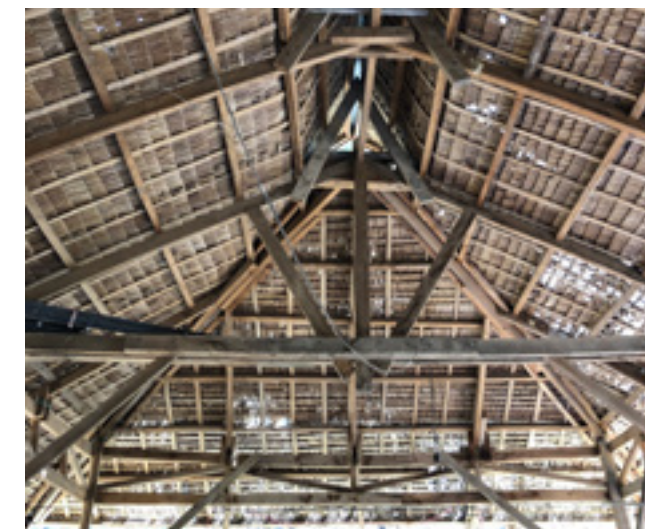
Figure 27 - Skews in longer beams
