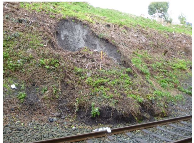
Figure 4. Examples of typical landslides on Irish rail network: a) on embankment, b) and c) on cutting
