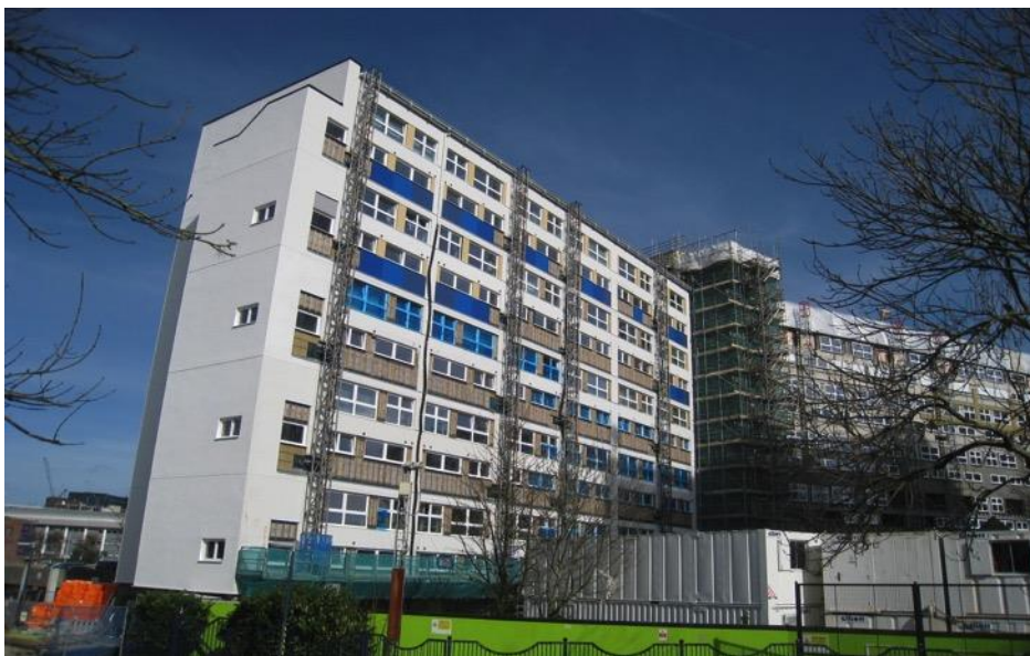
Block A Overcladding nearing completion: white externally insulated render (EWI) with blue coloured cladding – all low fire risk non-combustible insulation and limited combustible finishing materials
