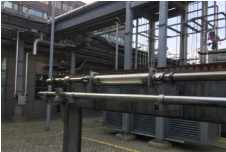
Figure 4.2: Photo of the inspection glass at the flowline of the SSL
