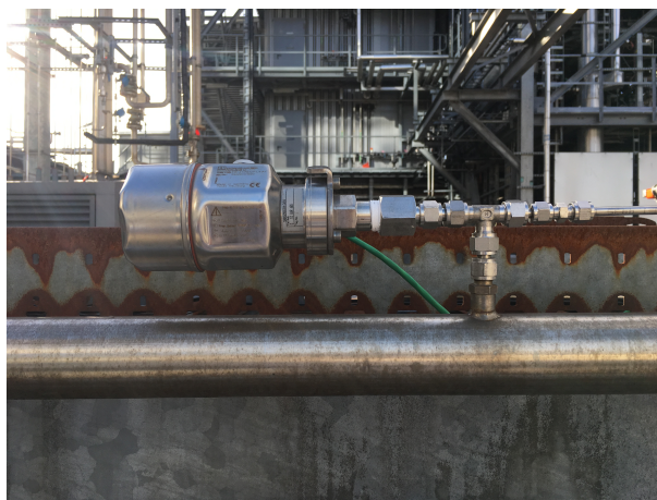
Figure 4.8: Pressure sensor PI-210 near the end of the flowline
