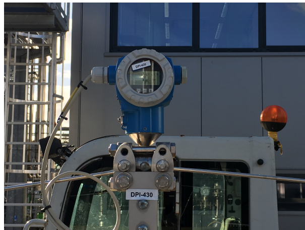
Figure 4.6: Differential pressure sensor DPI-430 along the flowline
