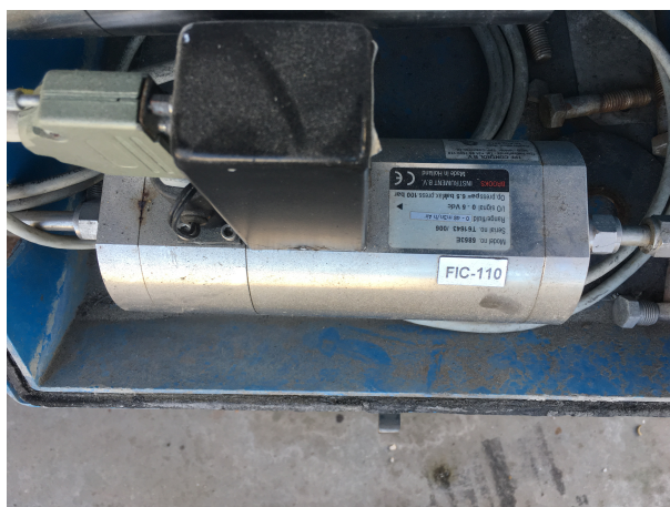
Figure 4.10: Volumetric flow meter of the air FI-110 with a low range
