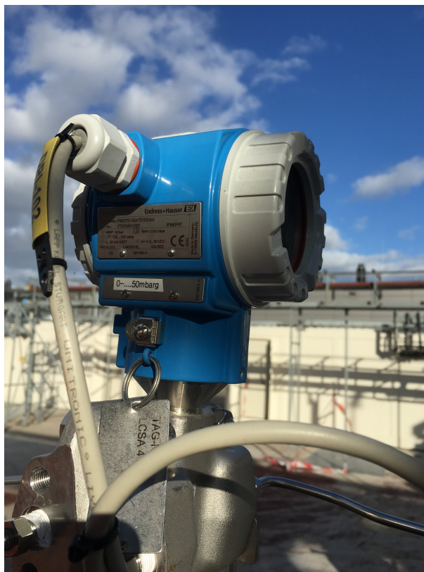
Figure 4.7: Differential pressure sensor DPI-102 near the end of the flowline
