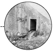
waste water outlet
