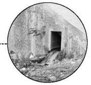
waste water outlet
