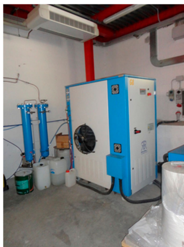
Figure 3. Electrolyzer G Series H0 3 supplied by Erredue Srl.
