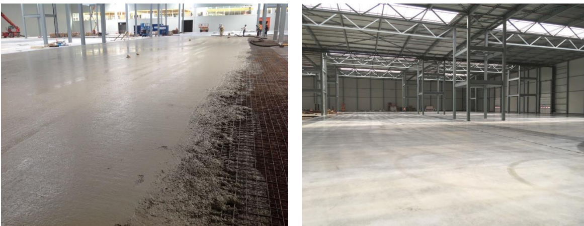
Figure 2.2 Industrial jointless concrete floor of the BIC Eindhoven hall being cast (left) and after hardening (right).
