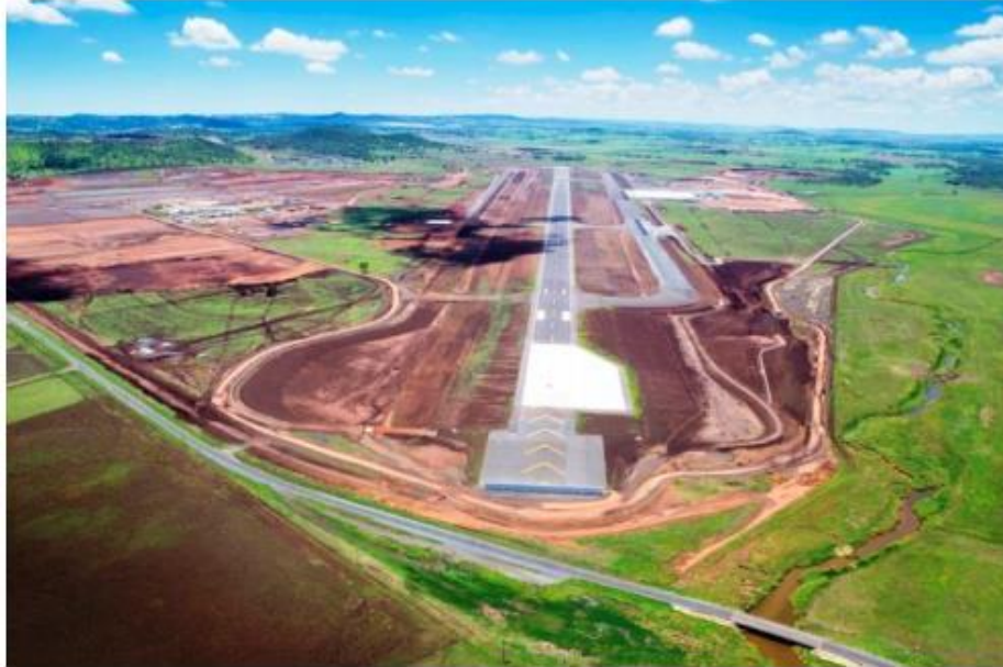
Figure 4.6 Aerial photograph of the completed pavement works at the Brisbane West Wellcamp Airport site (Glasby, Day, Genrich, & Aldred, 2015).
