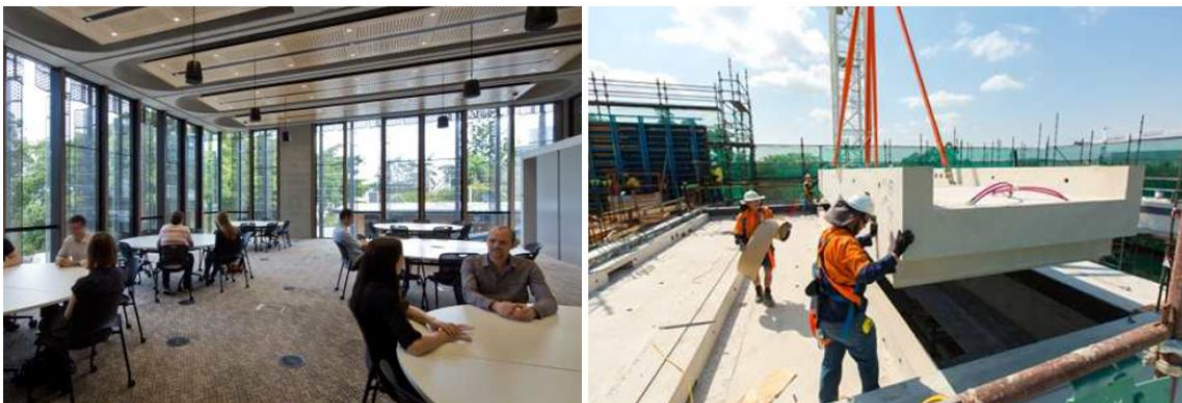
Figure 4.5 The Global Change Institute building of the University of Queensland (left) and the assembly of that building showing the geopolymer concrete floor beams (right) (Bligh & Glasby, 2013).
