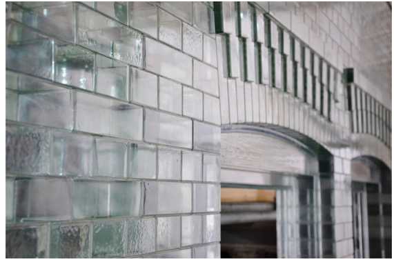
Fig. 1 View of the Crystal Houses, assembled from cast glass elements mimicking ceramic masonry. Derived from (Oikonomopoulou 2019)
