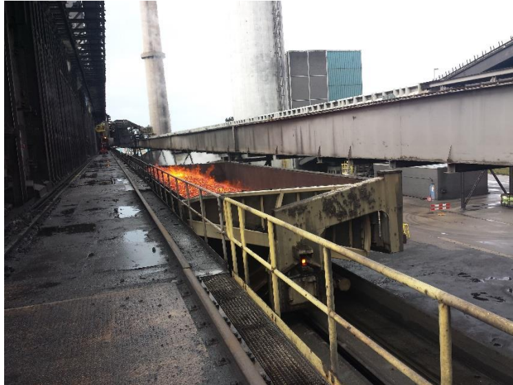
FIGURE 2.8 - QUENCHING CAR AT CGP 2, TATA STEEL IJMUIDEN
