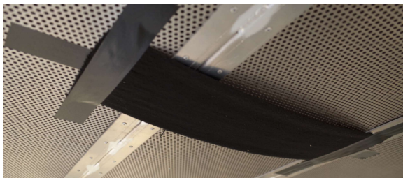
Figure 4.19: Black theatre-cloth attached to the fume hood to prevent reflections
