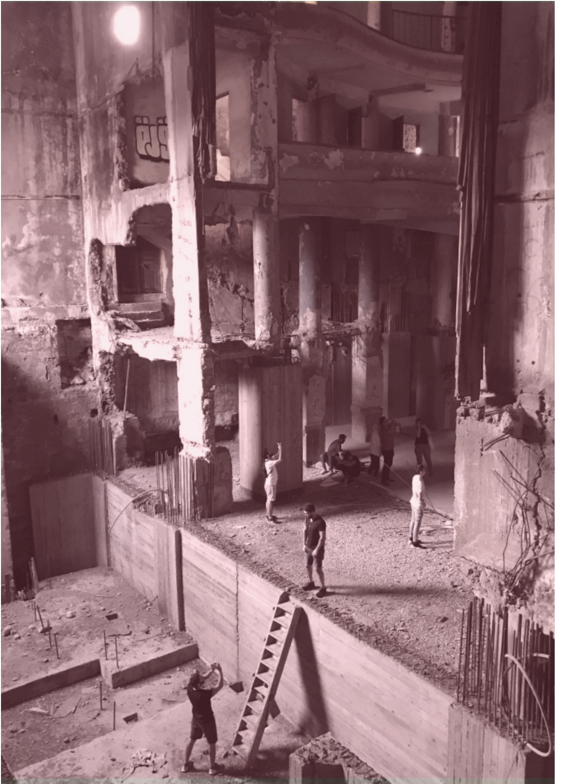
Figure: Picture of the Grand Theatre, heavily damaged by a history of catastrophes and municipal negligence.
