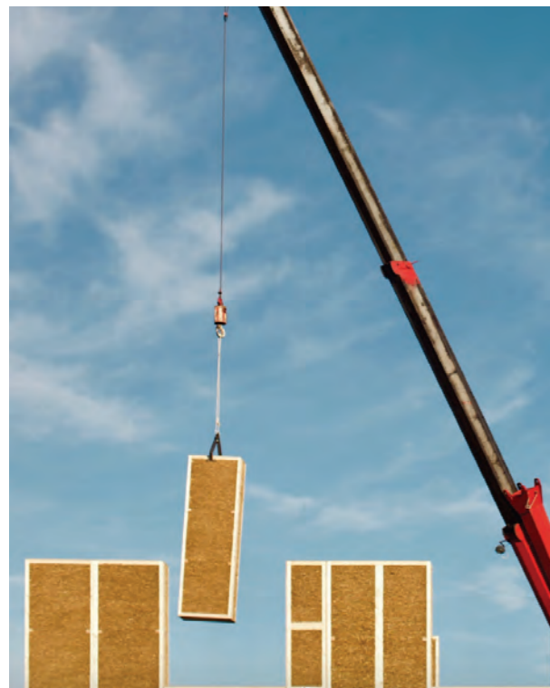
Fig. 47 Installing of Ecococoon's panels, a type of insulation made with straw Ecococoon, 2020
