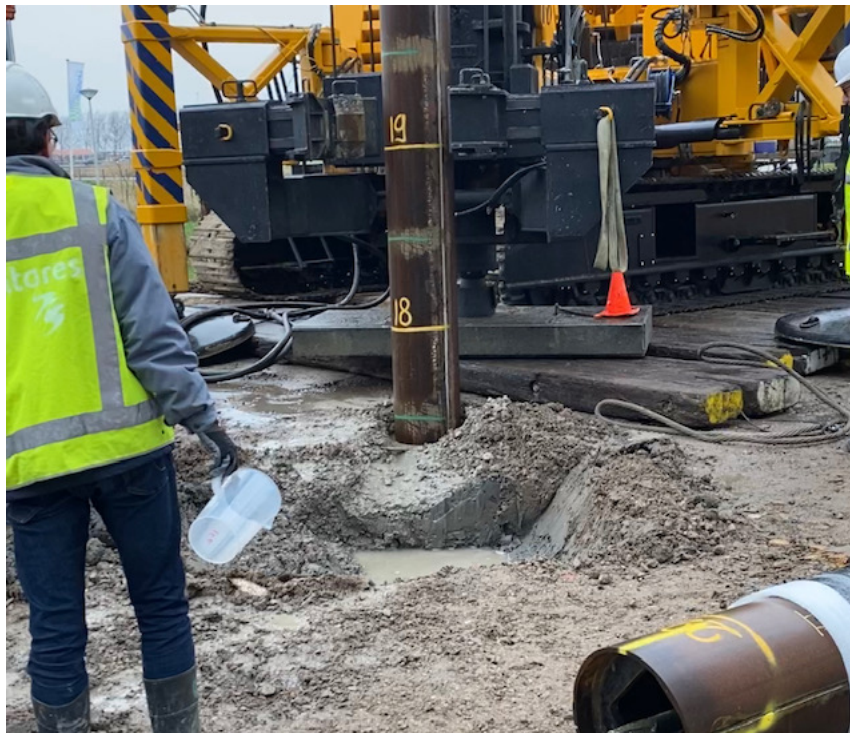
Figure 4.62: Grout collection during the installation of one of the Tubex piles at Thijsseweg. Outcoming grout would flow into the ditch, allowing for safe collection.
