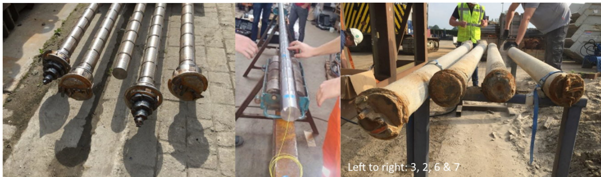
Figure 4.32: Left to right: pile tips and centre steel cylinder; strain gauges installed along steel cylinder; piles after extraction (NVAF 2019).
