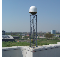
Figure 2.9: Station DLF1 in Delft is an example of a sensor station with good visibility, source: http://www.igs.org/igsnetwork/network_by_site.php?site=dlf1
