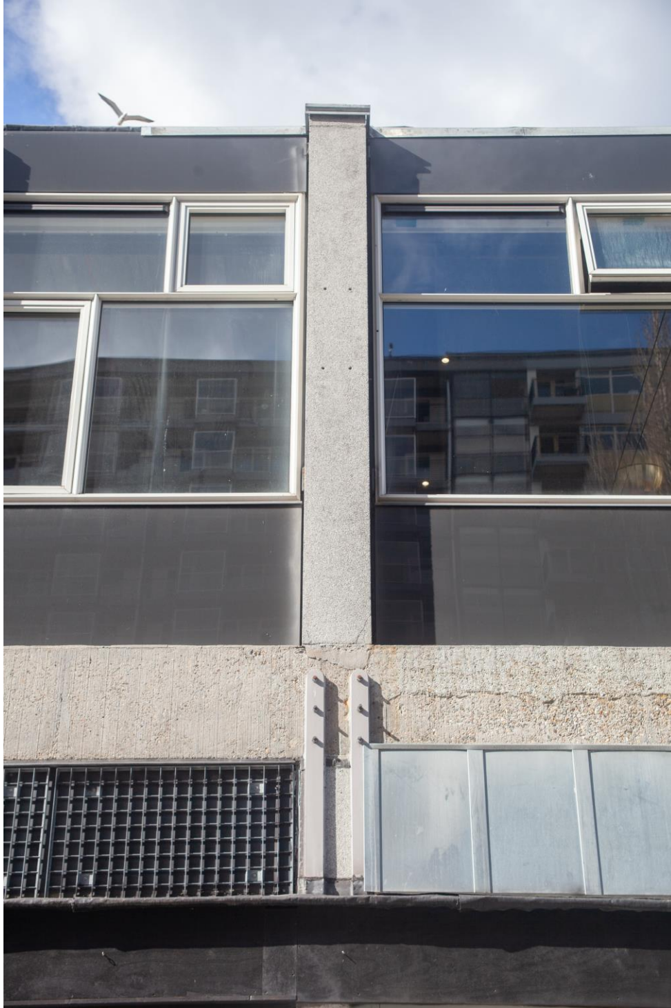
Figure 18 – The facades of the first floors show some signs of wear, with shops making adaptations over time. The concrete structure is clearly visible, along with steel beams and columns on the ground floor.
