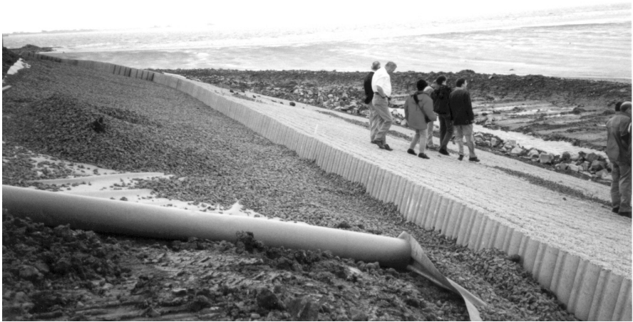
Granular filter and a geotextile under a Hydroblock revetment (photo H.J. Verhagen)
